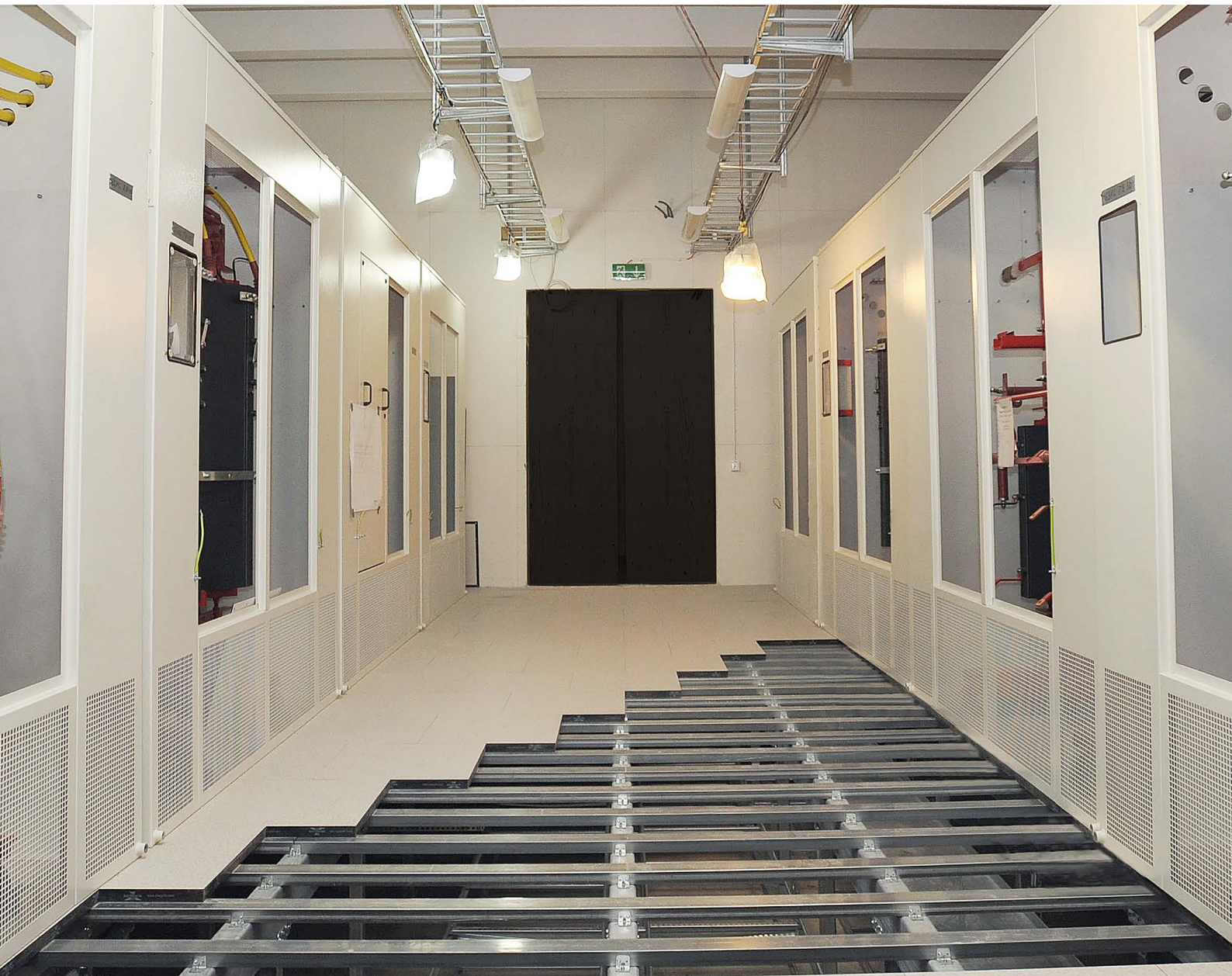
Transformer Room at Karolinska Hospital with reinforced Iso Floor Substructure supporting 16 Transformers with a total weight of 120 ton (265,000 Lbs).
