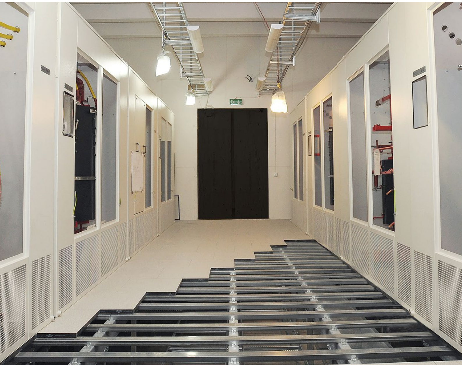
Transformer Room at Karolinska Hospital with reinforced Iso Floor Substructure supporting 16 Transformers with a total weight of 265,000 Lbs (120 ton).
